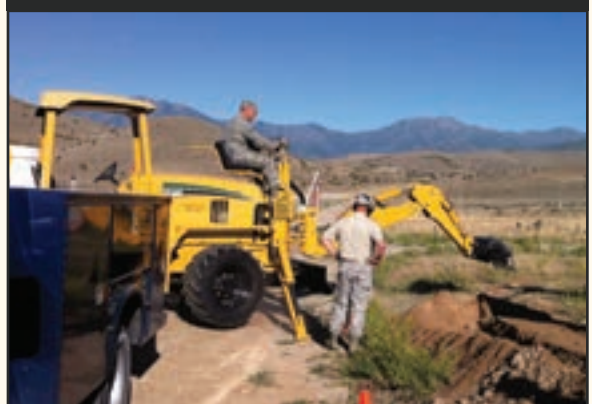
Army predeployment CST Training. Senior Airman Adam Farley completes a fiber installation project while deployed to the Persian Gulf. Gowen Field, Idaho, installation team. Members of the 130th work on a project to bury conduit for seven miles of fiber-optic cable to connect Camp Williams ranges.
